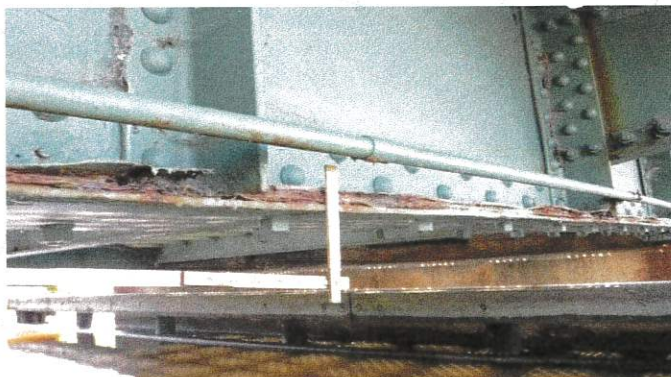
Active corrosion and pack rust on the bottom flange of the bascule girders
