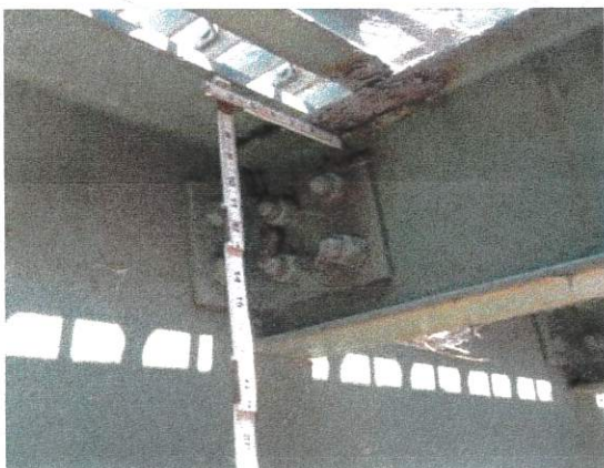
Active corrosion on a transverse deck stringer
